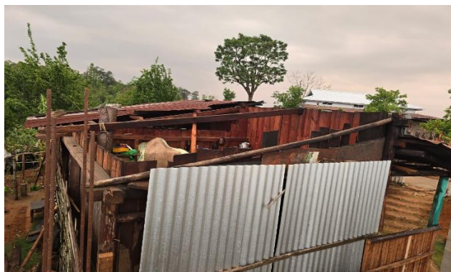
House damaged at Nongthyllep village under Mairang C&RD Block, Eastern West Khasi Hills District
